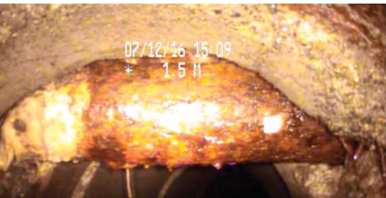
CCTV inspection showed several areas of concern in the sewers, including sections where water lines passed right through the sewer.
